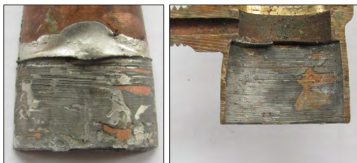
Figure 1: improperly Heated Solder Joint – Brush marks from mechanical cleaning (stainless steel brush inserted in power drill) still evident in soldered surface indicating inadequate heat in the tube surface leading to a lack of solder fill in the capillary space.
